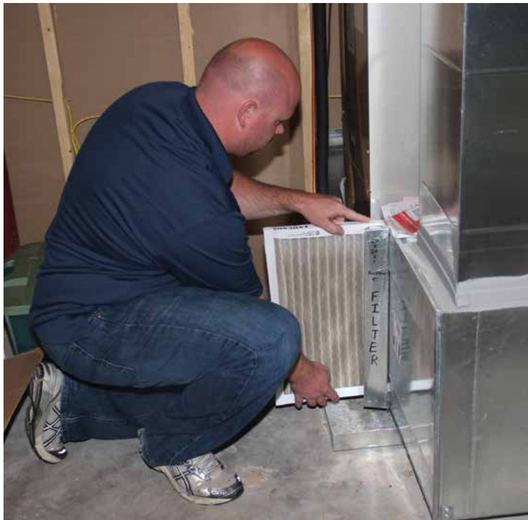
Changing your furnace filter at least twice a year is a great way to keep your system running as it should, and save on your energy bills. You can even get a furnace filter "whistle" that will give you an audible reminder when the filter is ready to be changed.
